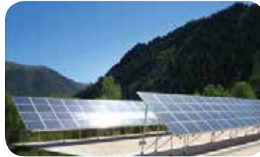
Solar panels at the City of Aspen water treatment facility.
