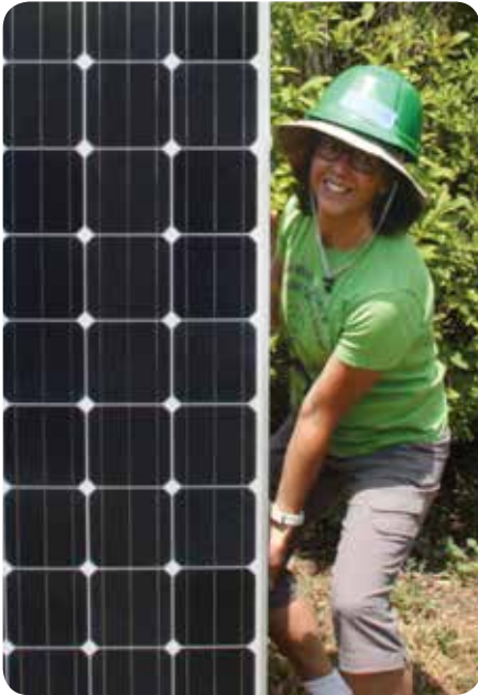
Mona Newton helps install a free solar array for an income-qualified resident.
