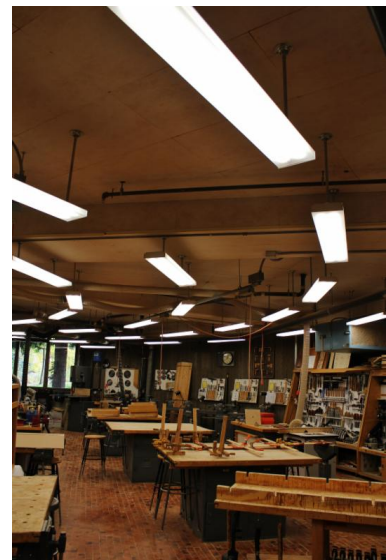
The new LED lights in the
